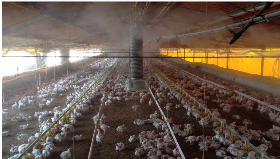
FIGURE 7. HIGH-PRESSURE MISTING SYSTEM IN A POULTRY BARN 46 .
