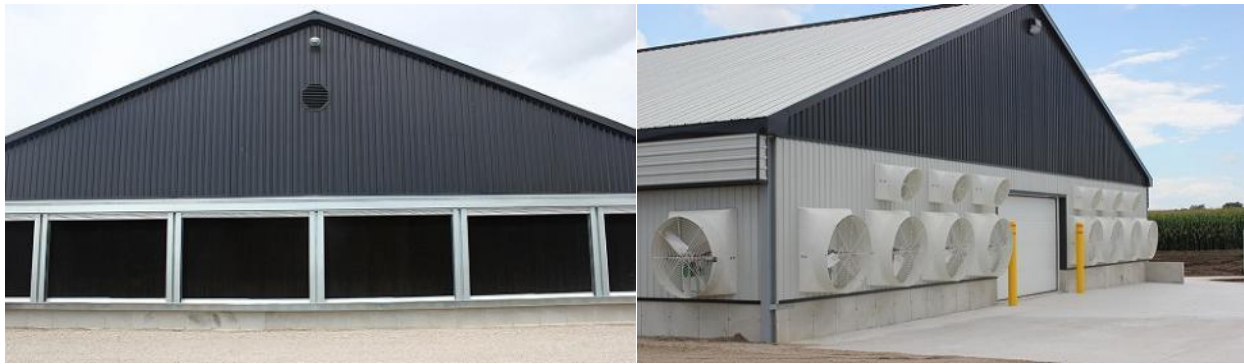
FIGURE 4. TUNNEL VENTILATION, INLET WITH EVAPORATIVE COOLING PADS INSTALLED (LEFT) AND EXHAUST FANS (RIGHT) 25 .
